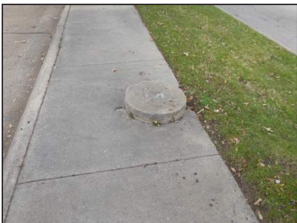
Figure 9-10 Tripping Hazard Example
