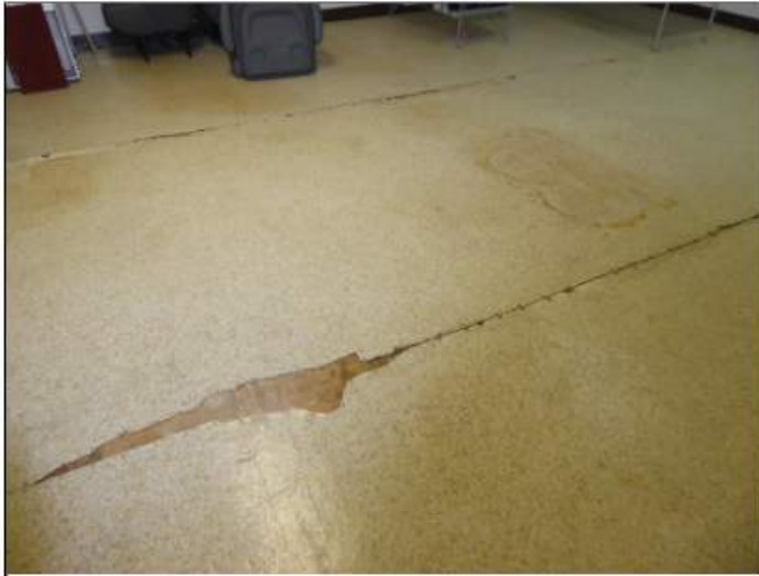
T-3 - Upstairs storage flooring in failing condition
