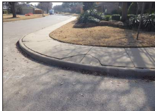
Figure 8-6 Example of a Non-Existent Curb Ramp
