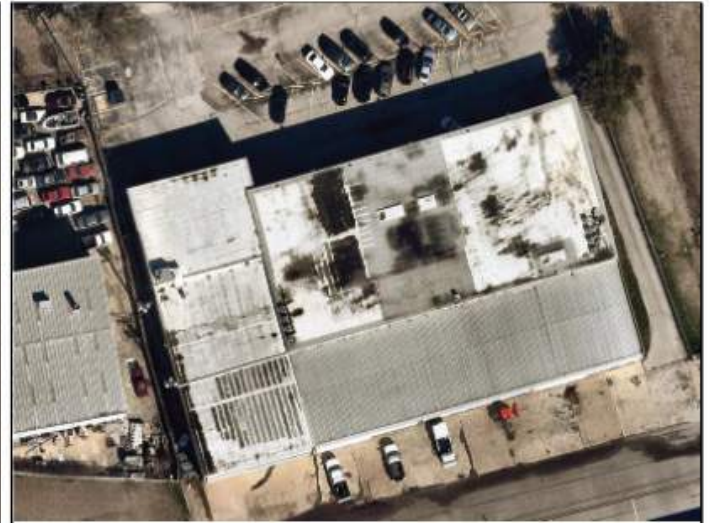
Wiley Post - Roof in failing condition
