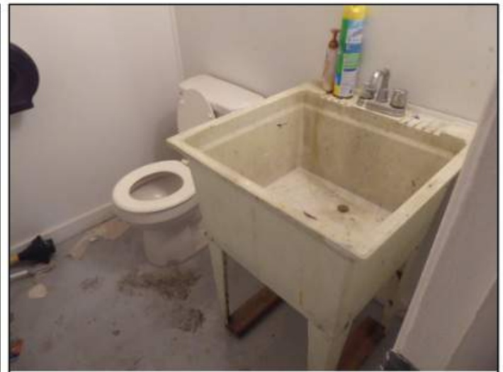
S-3 - Restroom assets in failing condition
