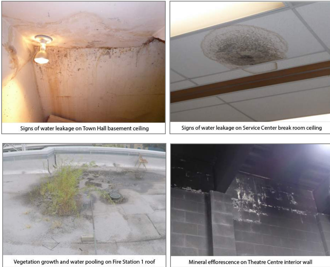
Figure 1-2 Failed/Failing (Condition 5) Building Assets
