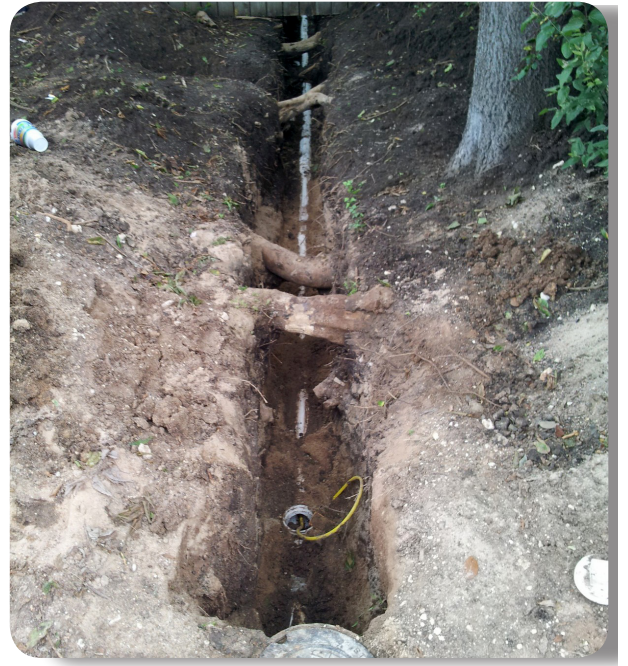
Change to tree roots are one of the top 5 causes of sewage overflows because the roots penetrate the sewage pipes.
