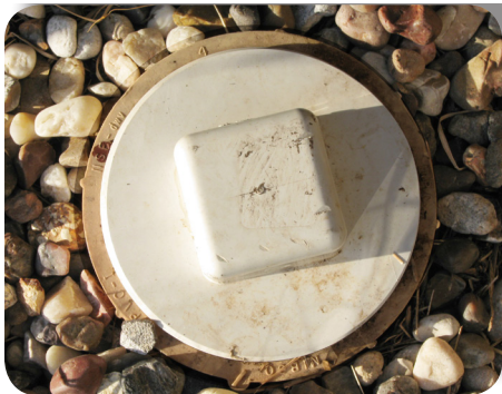
The property owner's cleanout cover is typically 4" in diameter.
