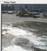
Wash out of solids/liquids
