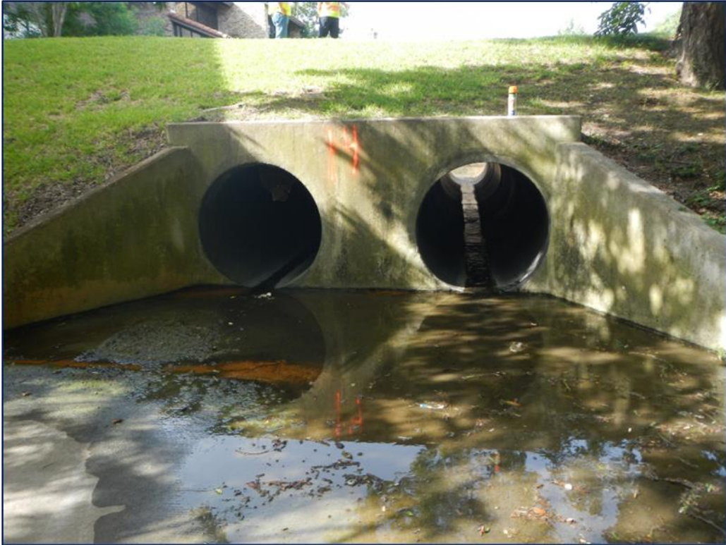
Outfall #14: 2 - 48" RCP that discharges from pond outlet (Outfall 13 above) to White Rock Creek Tributary 1.
