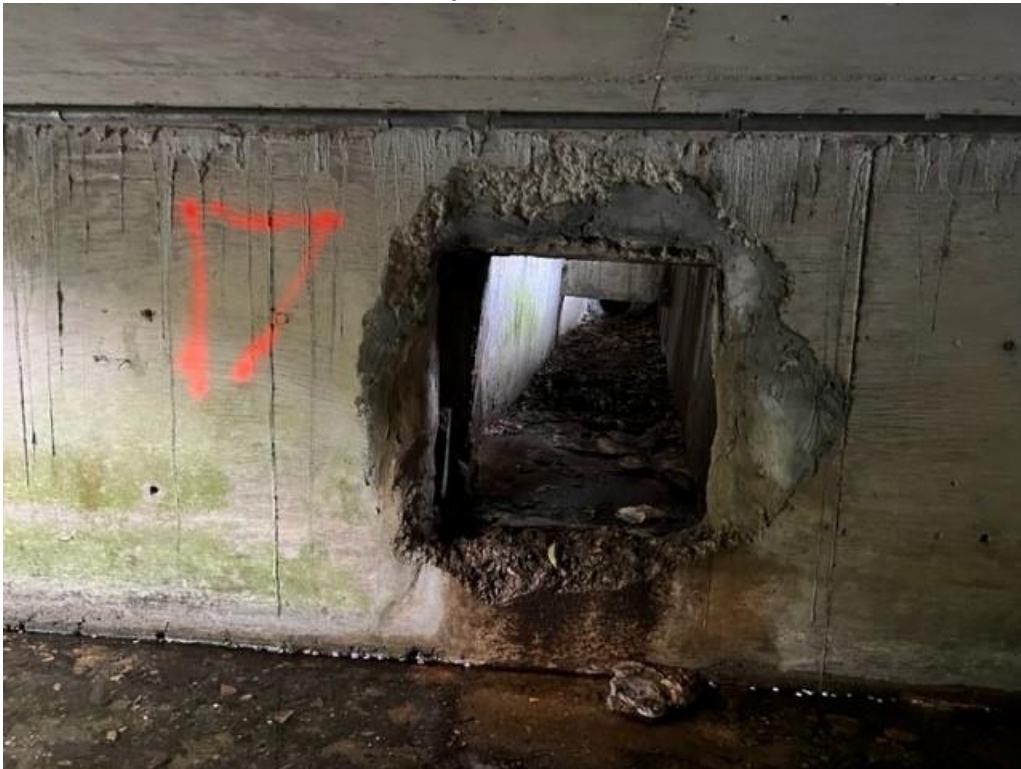
Outfall #17: 2' x 2.5' RCB that discharges into east side of boxed culvert under Oaks Dr.
