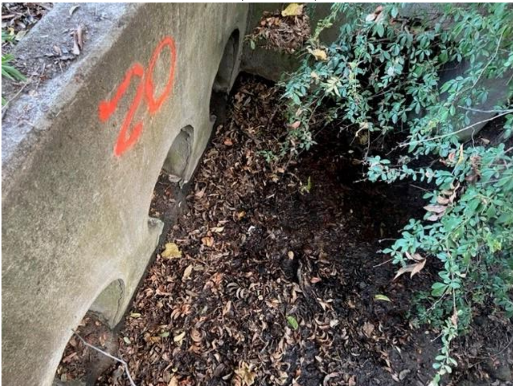
Outfall #20: 3 - 24" and 1 - 36" RCP from a closed system that discharges to a natural channel located near Winnwood Rd. and White Rock Creek Park.
