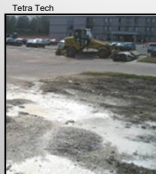
Wash out of solids/liquids
