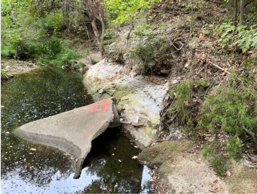
Outfall #21: 18" RCP from a closed system that discharges to a natural channel located east of Celestial Rd. Outfall has eroded and snapped at the joint.
