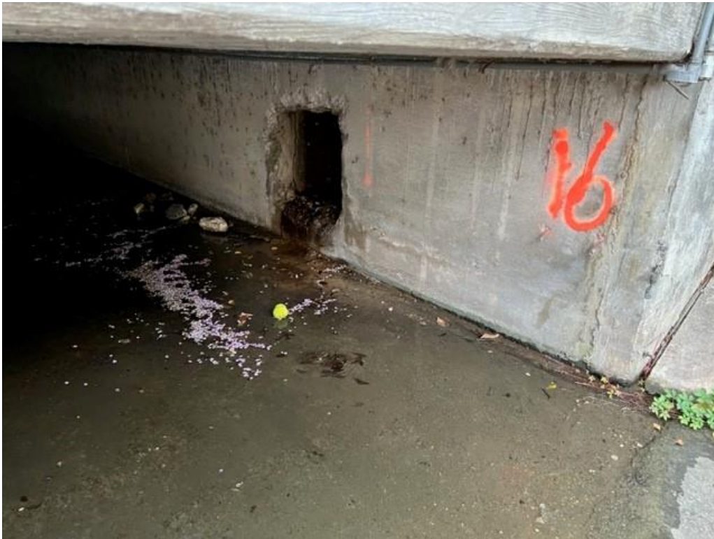
Outfall #16: 2' X 2.5' RCB that discharges into west side of box culvert under Oaks Dr.
