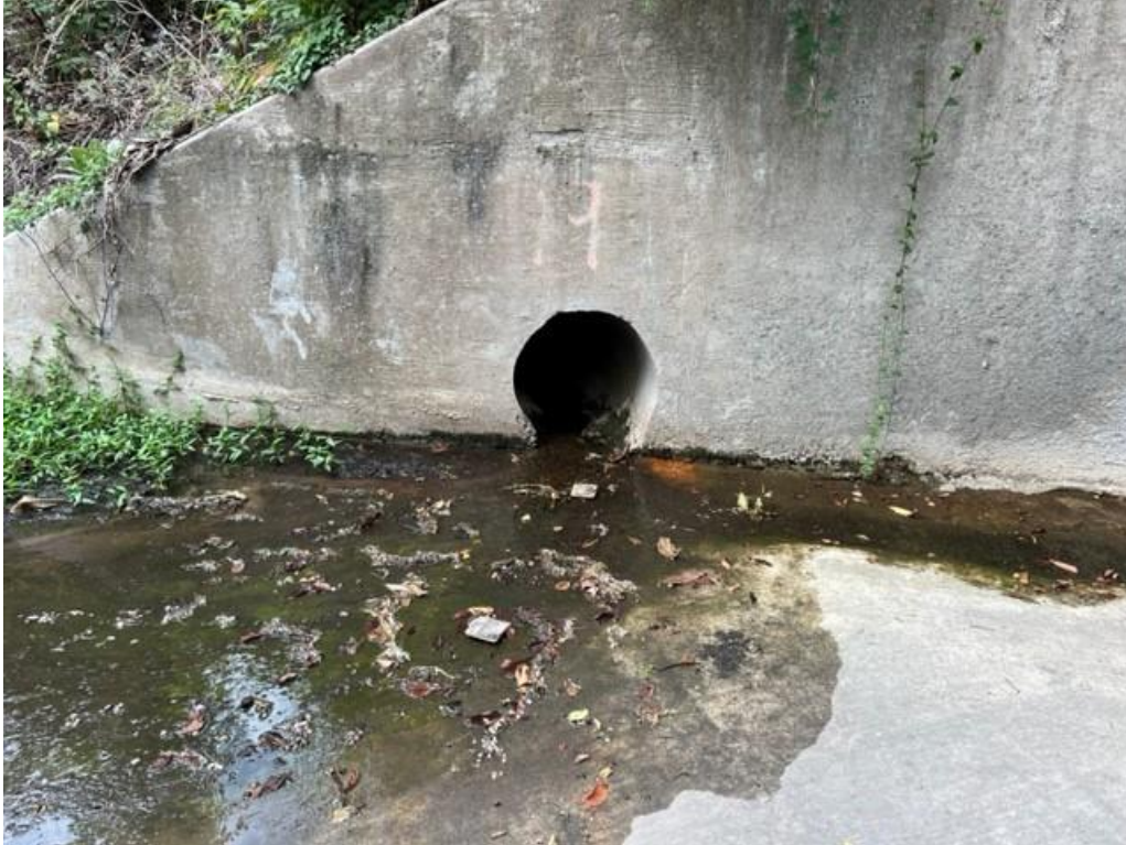
Outfall #19b: 18" RCP from closed system that outfalls into Winwood Park Pond Culverts (Outfall 19a).
