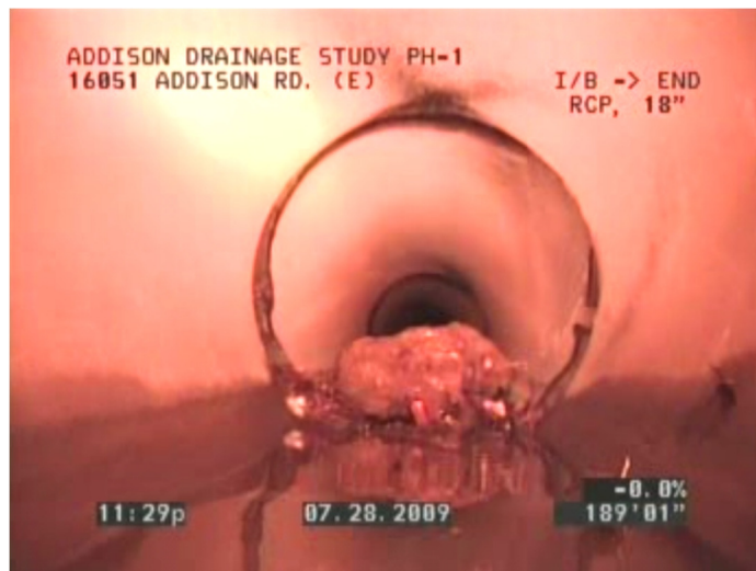
Photo V-1: CCTV Image of Problem Area in the Keller Springs Branch Basin
