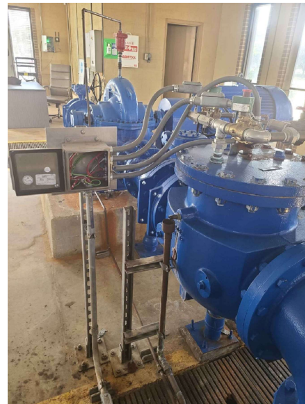
CONTROL VALVE PANEL PHOTOGRAPH A (TYP.)
