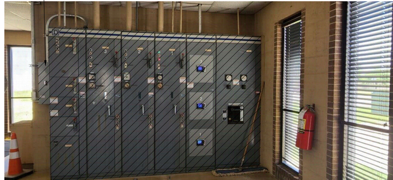
EXISTING PUMP STATION MCC PHOTOGRAPH B
