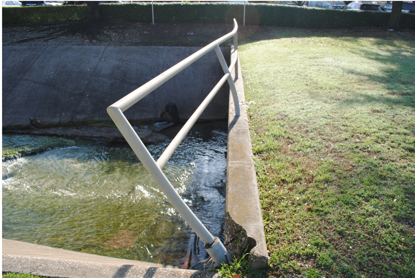
EXHIBIT 1: CONCRETE SPALL AT HANDRAIL ON SOUTH HEADWALL
